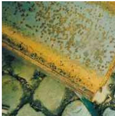
No. 18 Rust Spots Apparent
