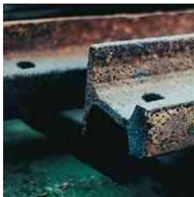
No. 20 Rust with pitting
