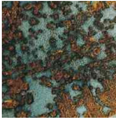
No. 19 Rust spotted
