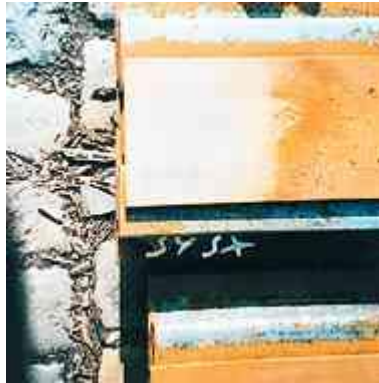
No. 15 Rust stained
