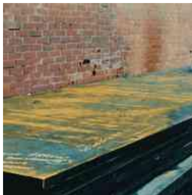
No. 16 Partly rust stained
